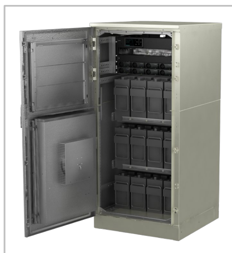
16kW Telecom system in outdoor cabinet
