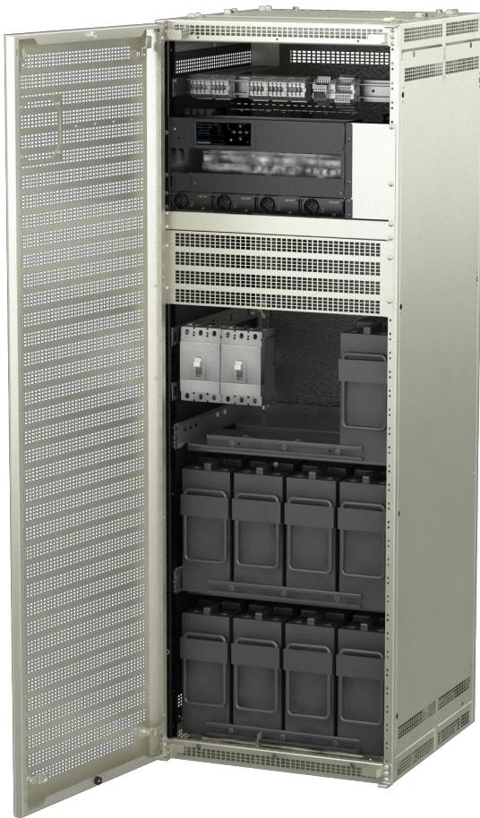
IBB system in FPC cabinet
